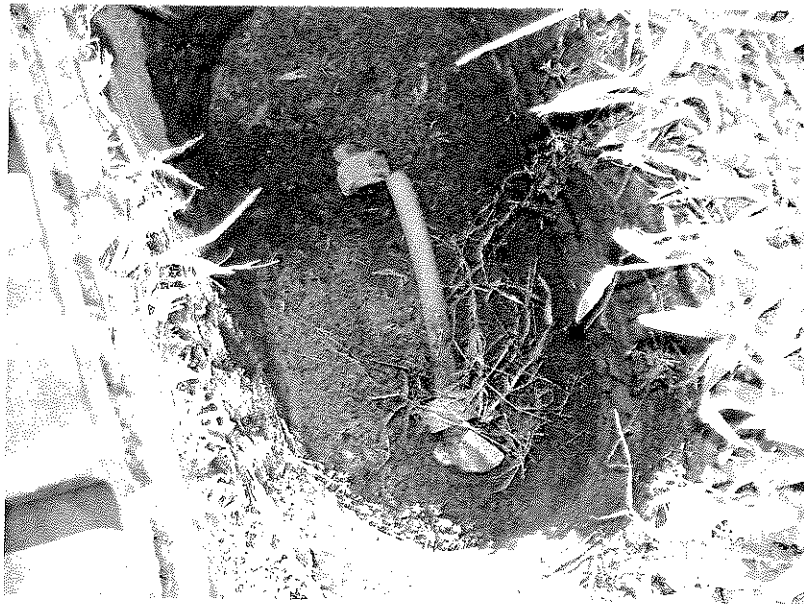
Straight Pipe of Water Meter with Garden Hose
