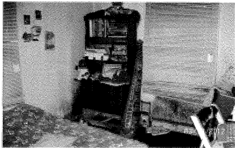
Moisture in the walls (Mold & Mildew)
